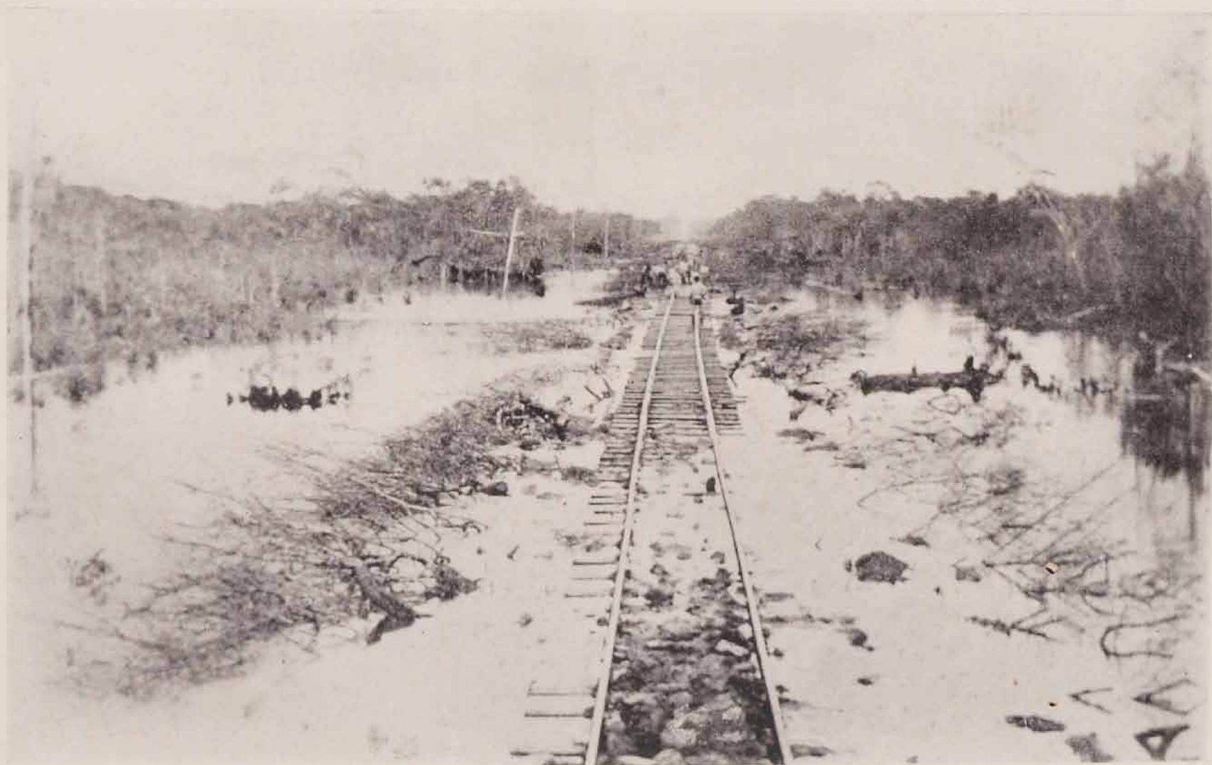
DIFFICULTIES OF RAILWAY CONSTRUCTION—RUNNING THE METALS THROUGH SWAMP ON CUT BRUSH FILLED UP WITH EARTH
