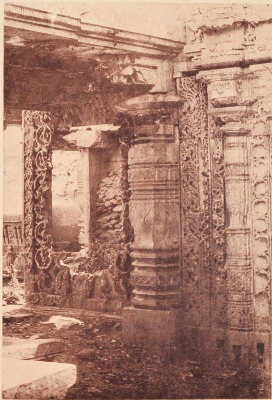
BANKAPUR: DAMAGED WINDOW IN THE TEMPLE OF ARVATTUKHAMBADA.
